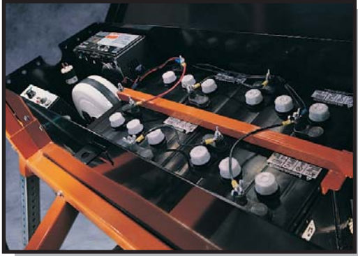
View of four, six volt deep cycle batteries
